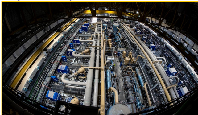
5000 tons of CryoPlant equipment
