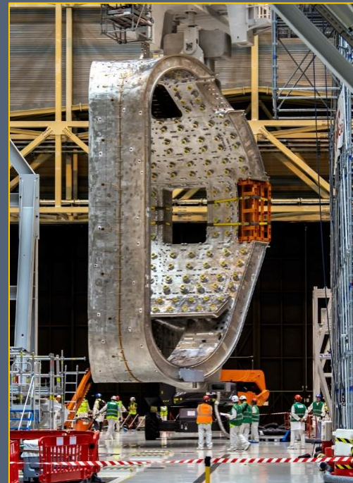
Vacuum Vessel Sectors: Dimensional non-conformities at field joint level
